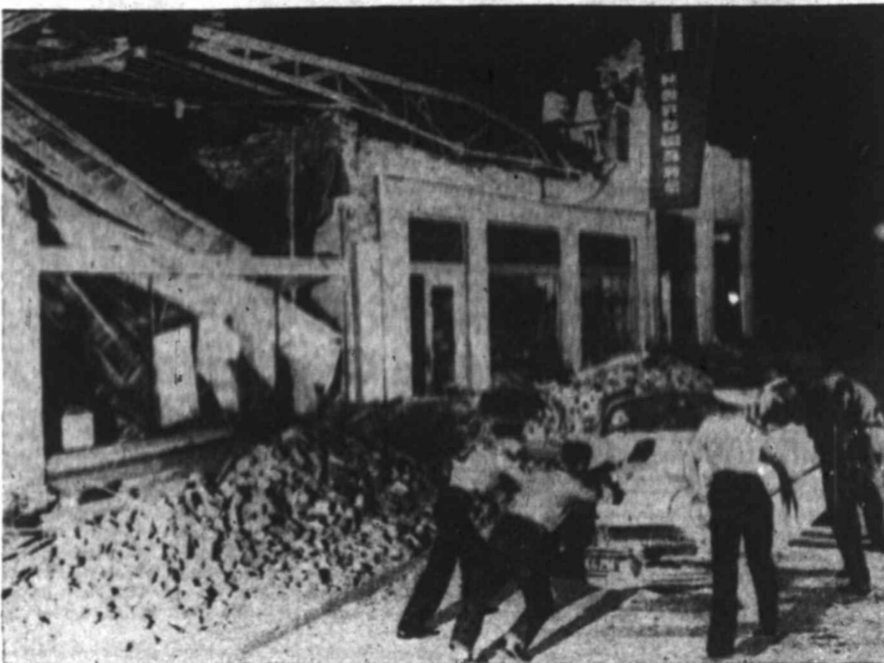
QUAKE DAMAGE—Salvage workers remove an already damaged automobile from the vicinity of a damaged building as the clean-up of Bakersfield, Calif., continues after the most recent of a series of earth shocks. The latest quake took a toll of two lives, injured 32, and caused property damage estimated at $20,000,000 or more.
