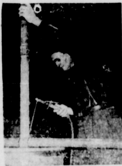
ATOM BOMB SHELTER ... Clarence Booth, of Lakewood, N. J., does some welding on the two-story atom bomb shelter he hopes to finish this summer. The 54-year-old inventor is confident that his structure, one story above ground and one below, will be virtually atom proof.
