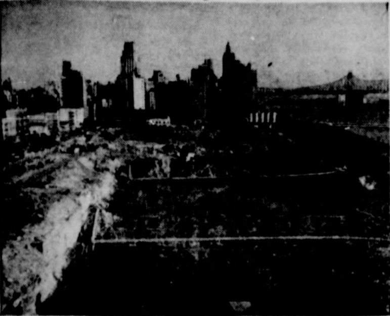
Excavations in the six-block site where the permanent headquarters of the United Nations are to be built in New York City are nearly complete. Meanwhile, U. N. signed a contract for $23,809,373 for the construction of the 39-story office building which will house its staff. The building is to be completed in the autumn of 1950.
