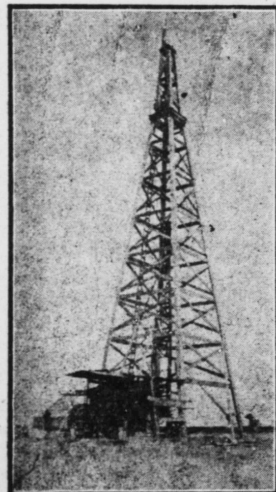
BLOCK 6, SECTION 6, BLOCK 2, H. & G. N. RY. SURVEY, REEVES COUNTY. DOWN ABOUT 900 FEET.
