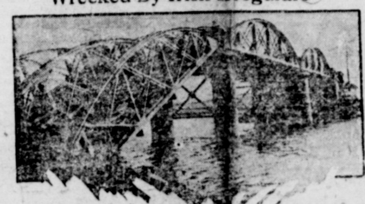
The Pota Bridge on the G. S. & W. railway between Queenstown and Cork, which was wrecked by Irish Irregulars to halt advance of Free State troops.
