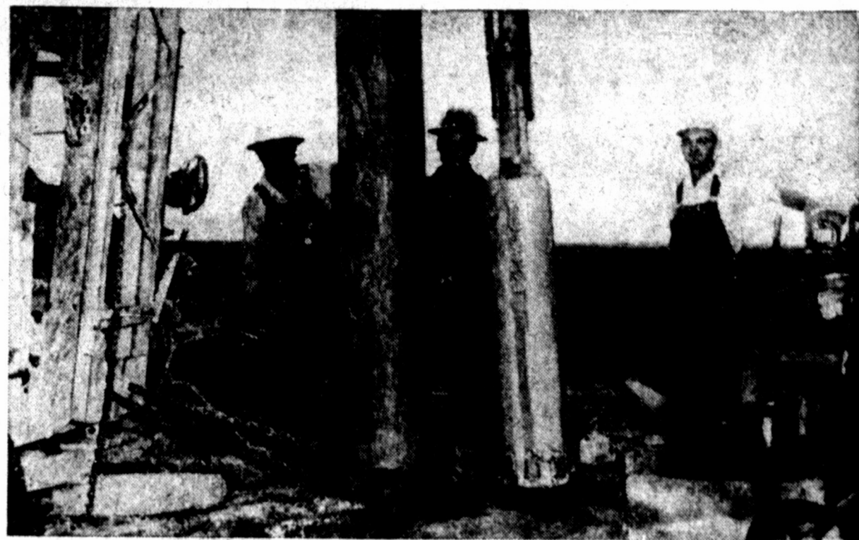
SHE CAVED IN —"One of the perils of irrigation farming is to have a well cave-in and cut off your water supply," said Grady Davis, right. Shown above is a crew re-working one of the two wells on the Davis farm. This particular well is located on the west side of his
