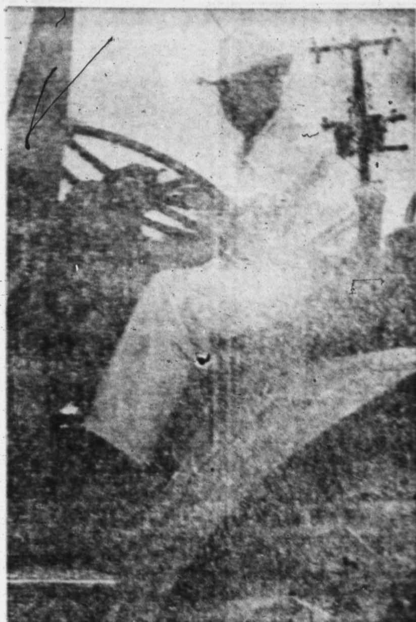
POWER ON WHEELS — John Swindall, a Tournapull operator for Ray Boswell Construction Company, will become a familiar figure around Brownfield before the widening project on Highway 51-62 is completed. Swindall operates a two-wheeled carryall machine that gouge out tons of dirt at one bite. (Staff Photo)
