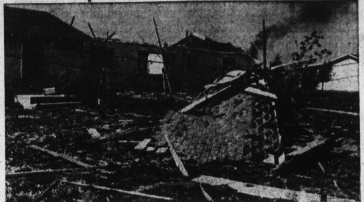
COMPLETE LOSS — One of the five tornadoes that danced around the Tokio Community last week unroofed the George Alexander home and heavily damaged the walls. Parts of the roof and walls were strewn about a mile across a pasture and road behind the home. Tornadoes also smashed at least four oil derricks in the area. (Staff Photo)
