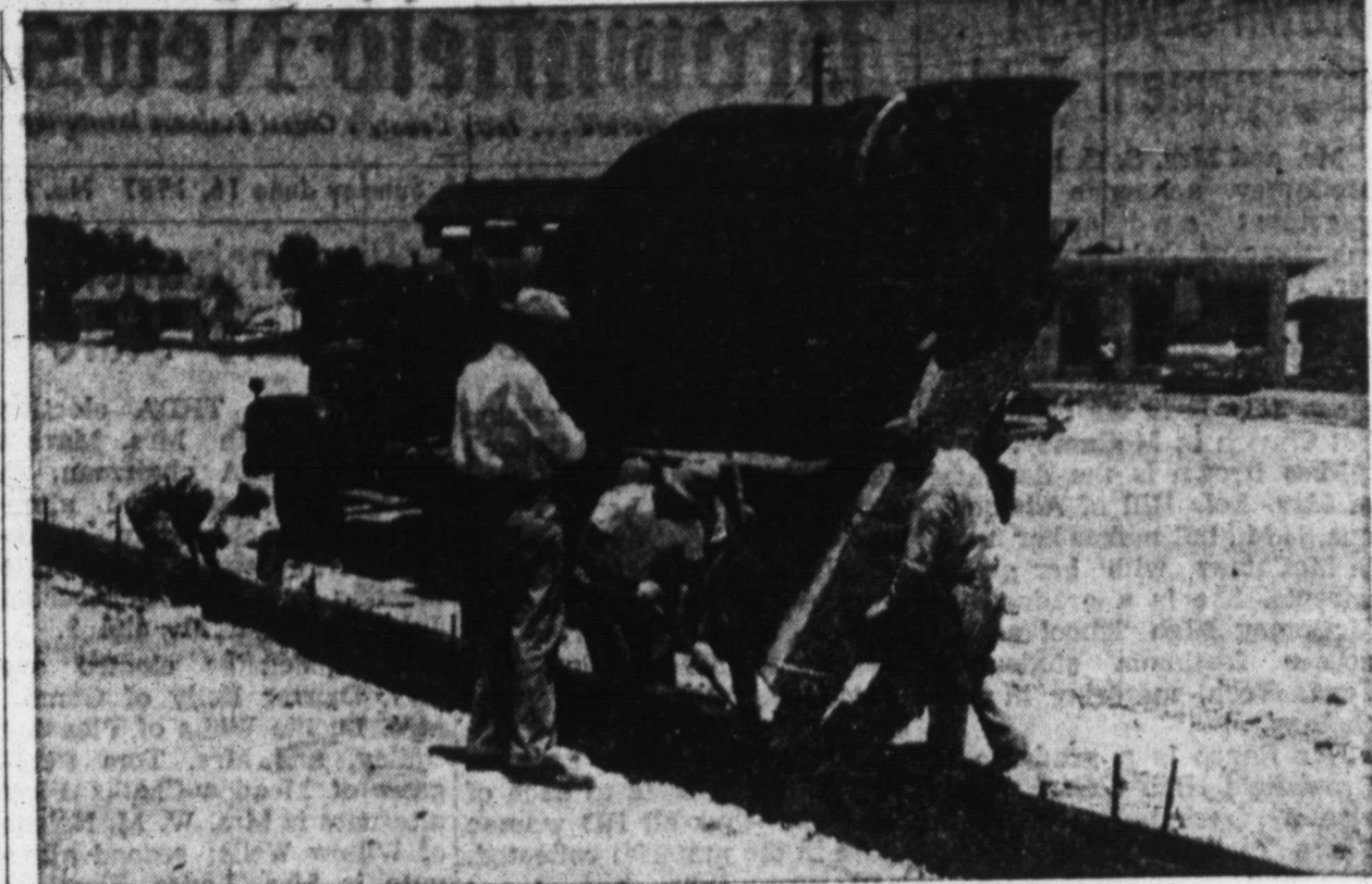
BEGINNING OF THE END — Construction on the road. Though the work marked a step toward completion, the work blocked many of the end this week as workmen rapidly poured concrete curbs and layed caliche along cross-streets and hampered travel in the area. (Staff Photo)
