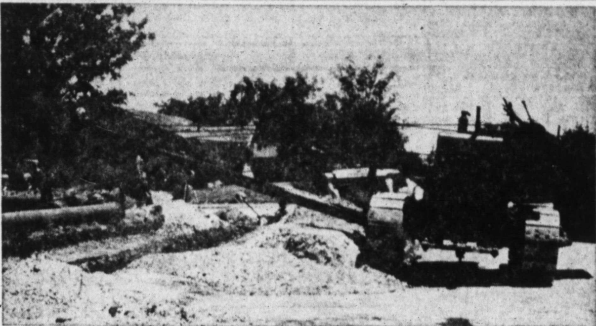
WATER LINES GOING IN — Final steps in laying service and supply lines in the toward completion of Brownfield's $270,000 southeastern part of the city. The expansion water expansion program were evident this is expected to be completed next month. week as Panhandle Construction Co. crews be- (Staff Photo)
