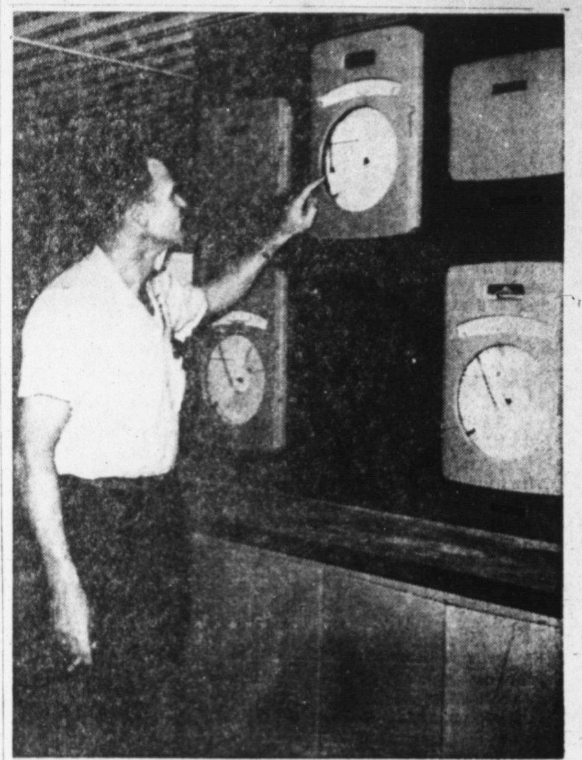
AUTOMATIC CONTROL PANEL — City Secretary Jake Geron checks a water level gauge on the control panel in the new pumping station just south of Coleman Park. The panel, which is controlled by mercury switches, shows the water level in storage tanks and automatically turns on well pumps to replenish them when the level drops to a specified point. (NEWSfoto)
