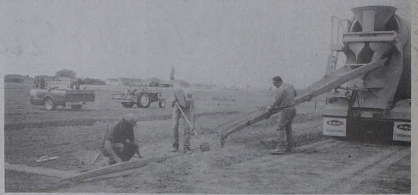
CONSTRUCTION BEGINS....Terry Copley and assistants Lynn Copley and Shannon Cochran, are shown pouring cement at a new project on West Highway 60. John Baca is reportedly set to build additional storage facilities there.
