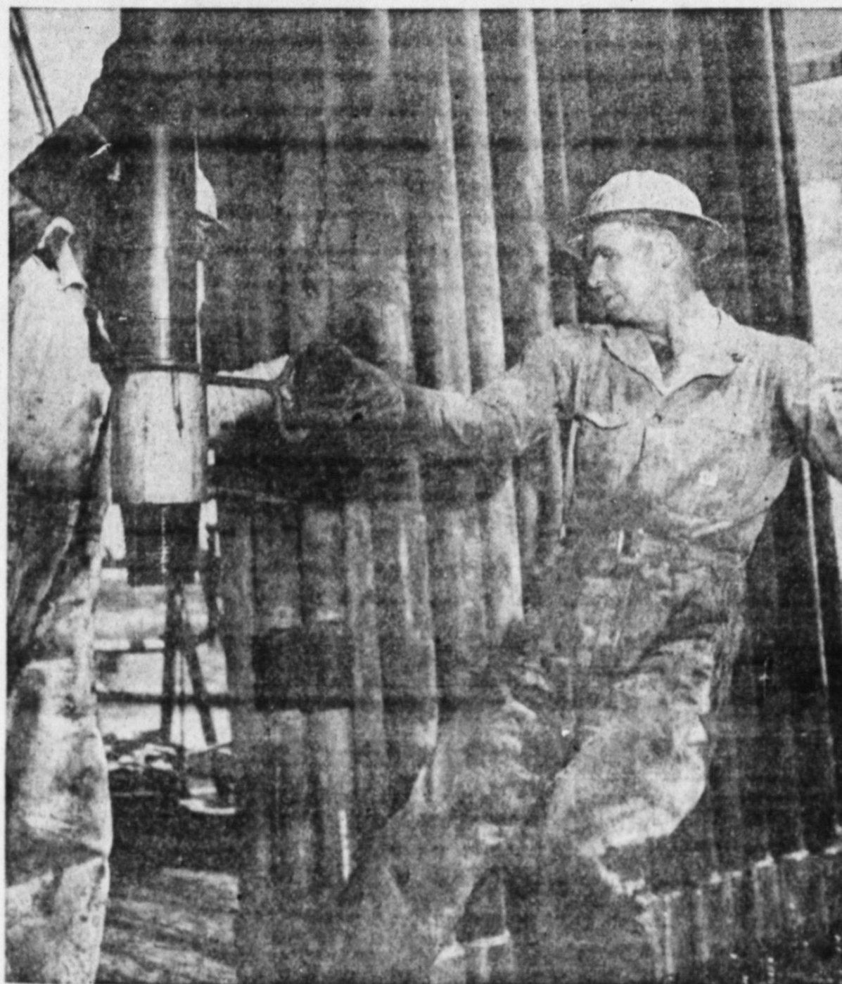
STAB THAT PIPE —Down she goes, and when this stand of pipe has reached the prescribed depth—then, what will it be? Maybe a gusher, maybe a dry hole . . . but you will always know that men such as these are constantly at work seeking new "pay" and developing new fields. Much credit is due these men—"the roughnecks," who work around the clock, seven days a week to bring in more oil . . . "Everyone benefits from Oil."
