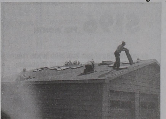
ROOF WORK--- Several crews of roofers have been spotted on rooftops around town for the past couple of weeks. L.V. Pearson, Dennis Adams and Clyde Brown were found at work on the Terry residence on Columbia Street.
