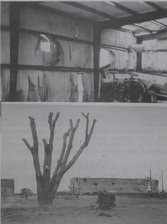
BARN DAMAGE..... Noel White's metal barn, on the old Goodwine place just south of Friona, was bombed by 55-gallon barrels during the June 2 tornado. The barrels had been stored in the rear of J&H Equipment. Some were also found on the McLellan property across Highway 60. Top photo shows the inside of the barn, with the outside shown at bottom, with holes evident. (Photos by Ron Carr)
