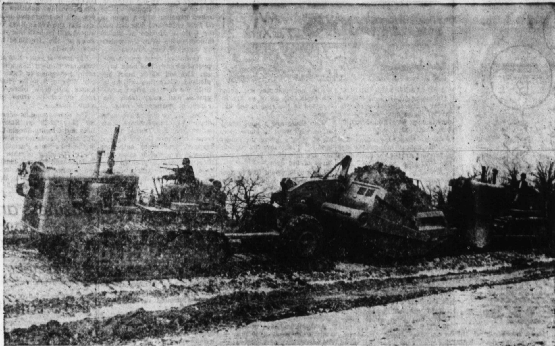
A REAL PAYLOAD — Proper slope loading scraper operations are demonstrated during one of the Heavy Construction Equipment Operators Schools conducted at Texas A. and M. College by the Engineering Extension Service.
