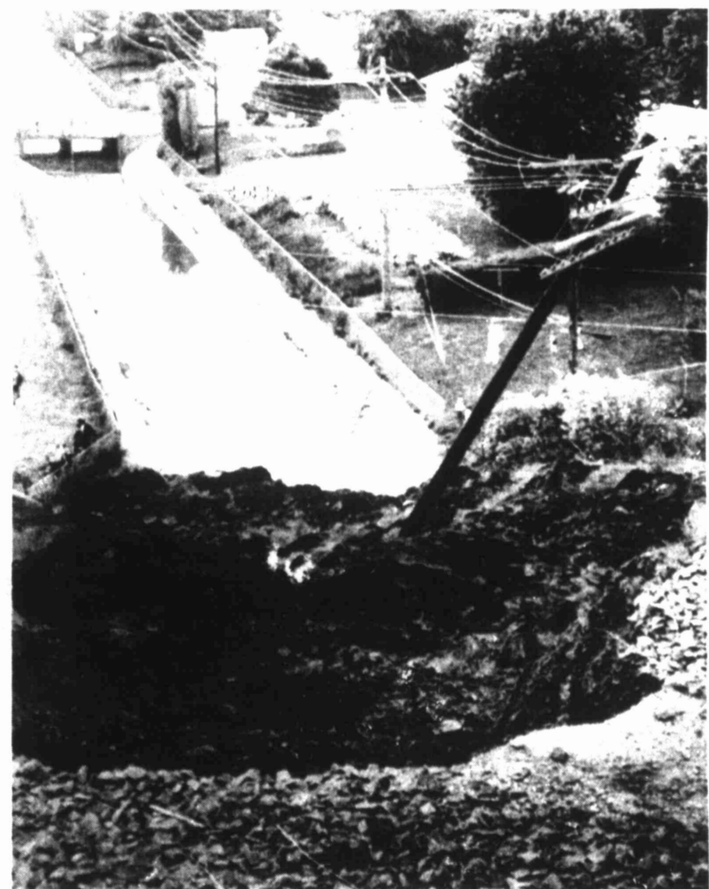
MUDSLIDE — Heavy rains the past two weeks are blamed for the collapse of a 125-foot embankment beneath Union Pacific Railroad tracks in West Omaha Sunday. This view from atop the embankment shows the tons of debris spilled into Hell Creek below. UP officials say the vibration of passing trains combined with the rains to collapse the embankment.
