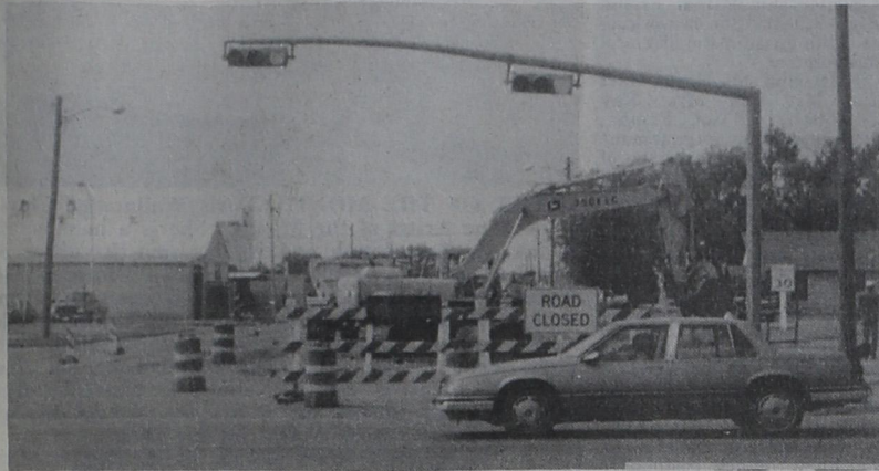
WHERE IS MAIN STREET?.....Work began with a vengeance this week on Friona's Main Street as the Texas Highway Department began remodeling sidewalks and curbs from Highway 60, above, to 5th Street on the south. Estimated completion is October. (Ron Carr Photo)
