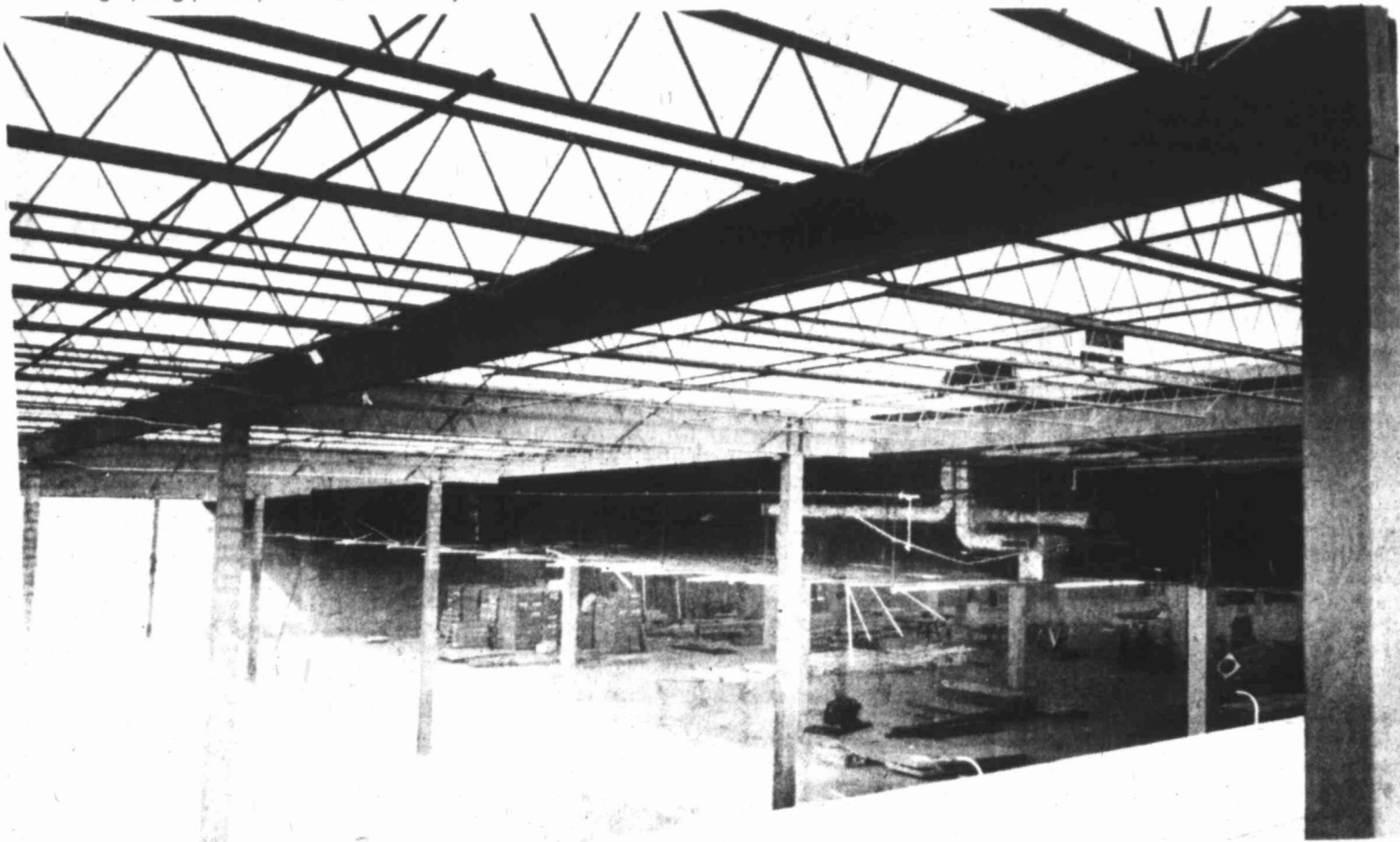
CONSTRUCTION UNDER WAY — Wal-Mart Discount City, a new discount store which will open in Big Spring in late summer or early fall, is under construction now at Coronado Plaza. The new store will be housed in what was once Thornton's Department Store. Several hundred feet of new store space is being added on to the new facility.
