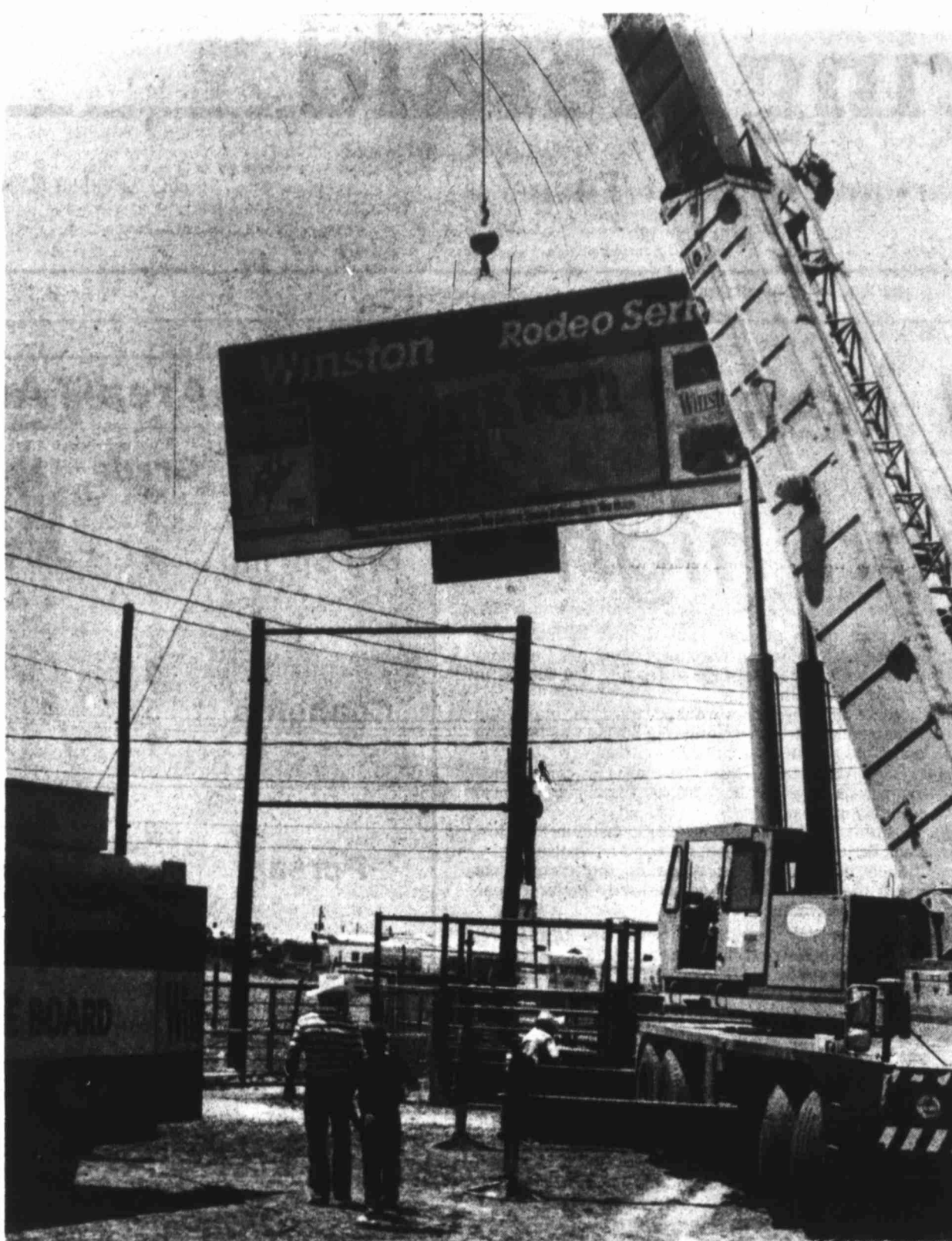
A SCOREBOARD FOR THE RODEO — Construction workers place a 2,500-pound computerized scoreboard atop a support Monday at the Big Spring Rodeo Bowl. The scoreboard, one of five used by the Winston Rodeo Series of the R.J. Reynolds Co., is 10-foot by 28-foot and is valued at $90,000. Winston chooses 40 rodeos in each year for the scoreboard, according to Ron Canaster, who supervised the work yesterday. The scoreboard keeps time, gives scores and can display messages and pictures. Cathey Construction of Big Spring worked on the installation.
