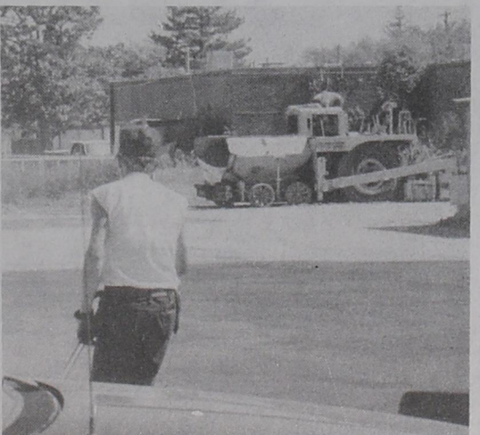
DONUT IMPROVEMENTS... Customers of Pappy Jack's Donuts will be delighted with the new asphalt paving on the parking lot and drive thru. Building owners Bill and Carol Ellis are making the improvements with Bermea Construction of Friona. (Ron Carr Photo)
