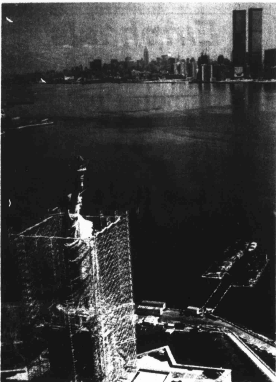
LIBERTY CAGED? — Scaffolding rises around the Statue of Liberty as part of a $30 million renovation project of the aging monument in New York Harbor.
