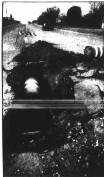
BIG SPRING — A road barrier sits fallen into the pit it is supposed to be guarding cars from along East Sixth Street. The pit was dug to fix one of the 107 broken water lines in Big Spring.
