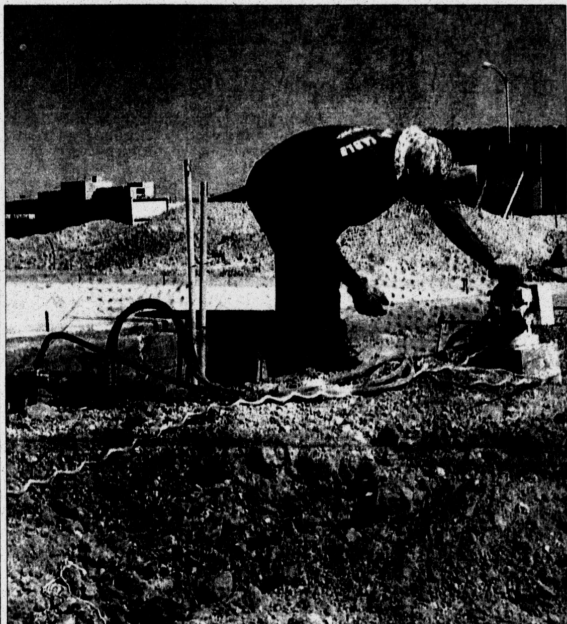
Lorezo Acosta, an employee of Larry Snyder and Co. of Missouri, works on the foundation of the Knollwood Apartment Complex, which is under construction at the intersection of FM 700 and Martin Luther King Boulevard. Construction is expected to be completed by early October, a company official said.
