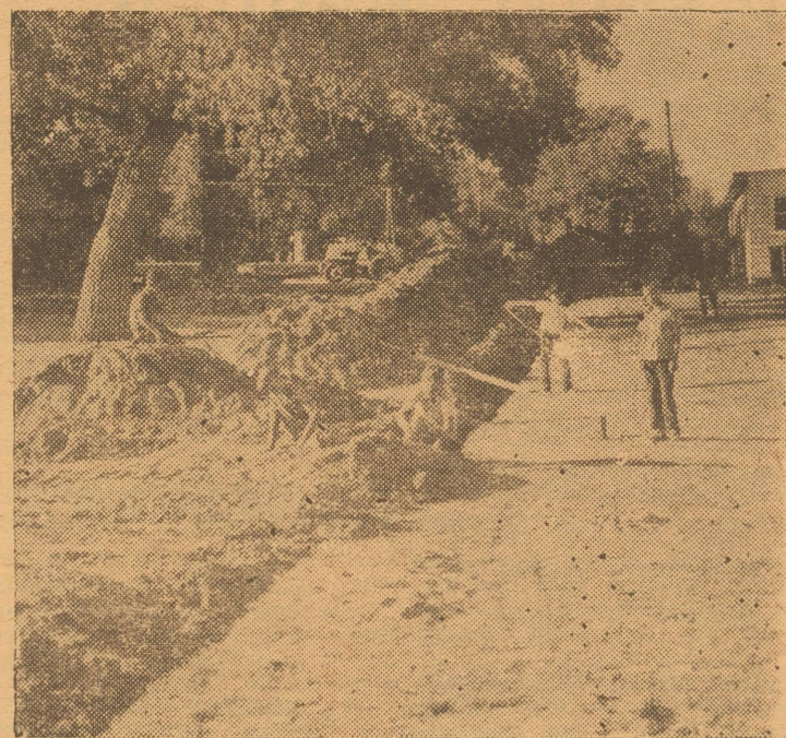
Boys' Ranchers lay 8-inch tile which connects the 26 buildings at America's First Boys' Ranch, Amarillo, Texas, to a central disposal unit. The new system will eliminate the many septic tanks at the Ranch which require frequent cleaning and will provide for future buildings.
