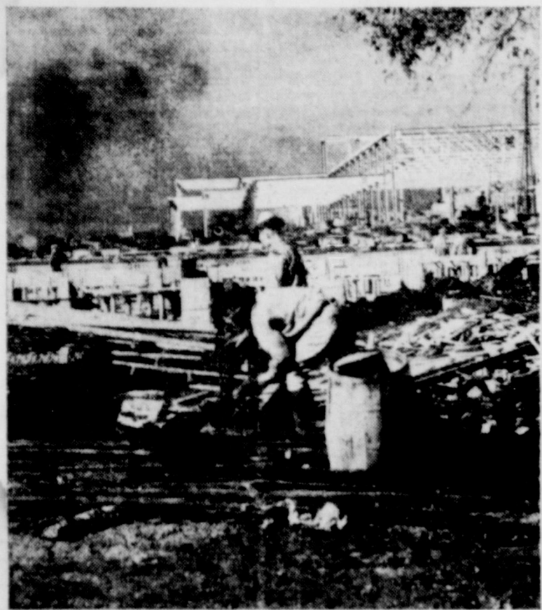
The steel frame of the $140,000 Livestock Building No. 2 for the Texas Centennial Exposition at Dallas can be seen above as it rapidly takes form. With the $269,000 Livestock Building
