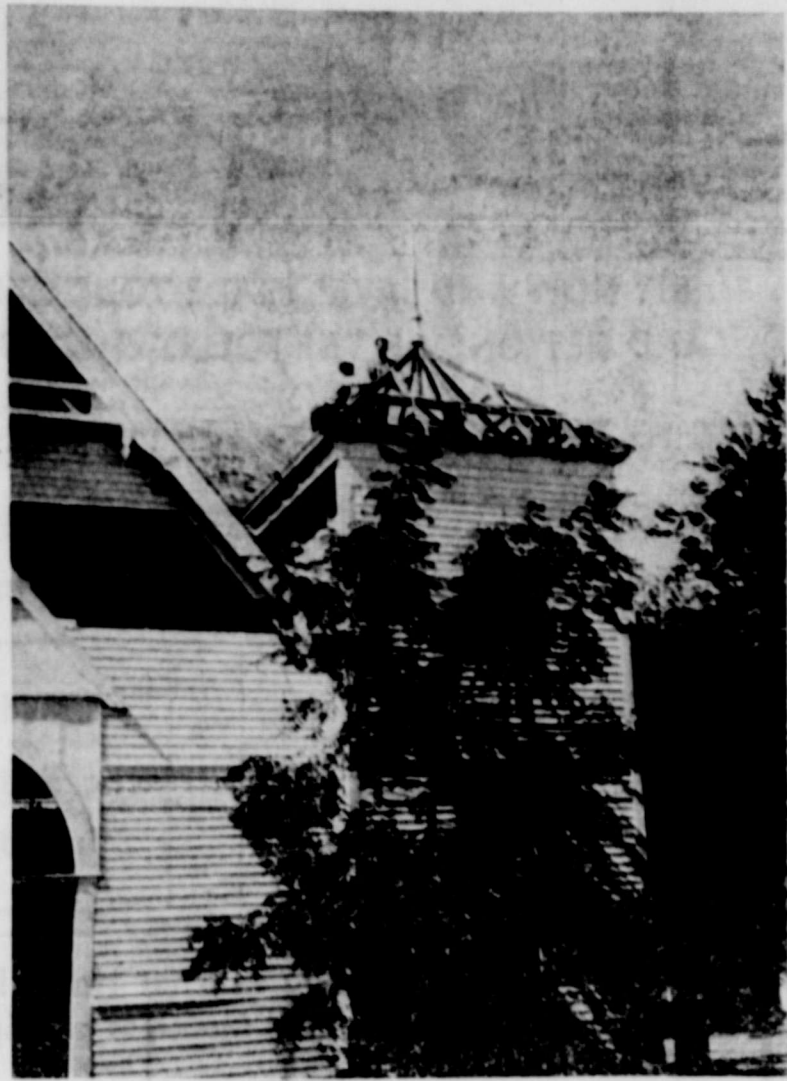
LANDMARK RAZED —One of Hico's oldest landmarks, First Baptist Church, is in process of being razed to make way for a new, modern building. This shot of the demolition
