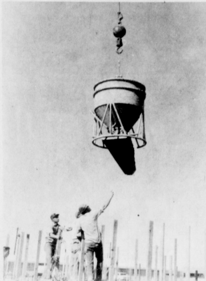
CEMENT WORK. . . Pouring of cement began in earnest at the new Friona State Bank site on Monday, as the contractor used a giant steel container and a crane to get the cement to the critical places. In these pictures, action shows the
