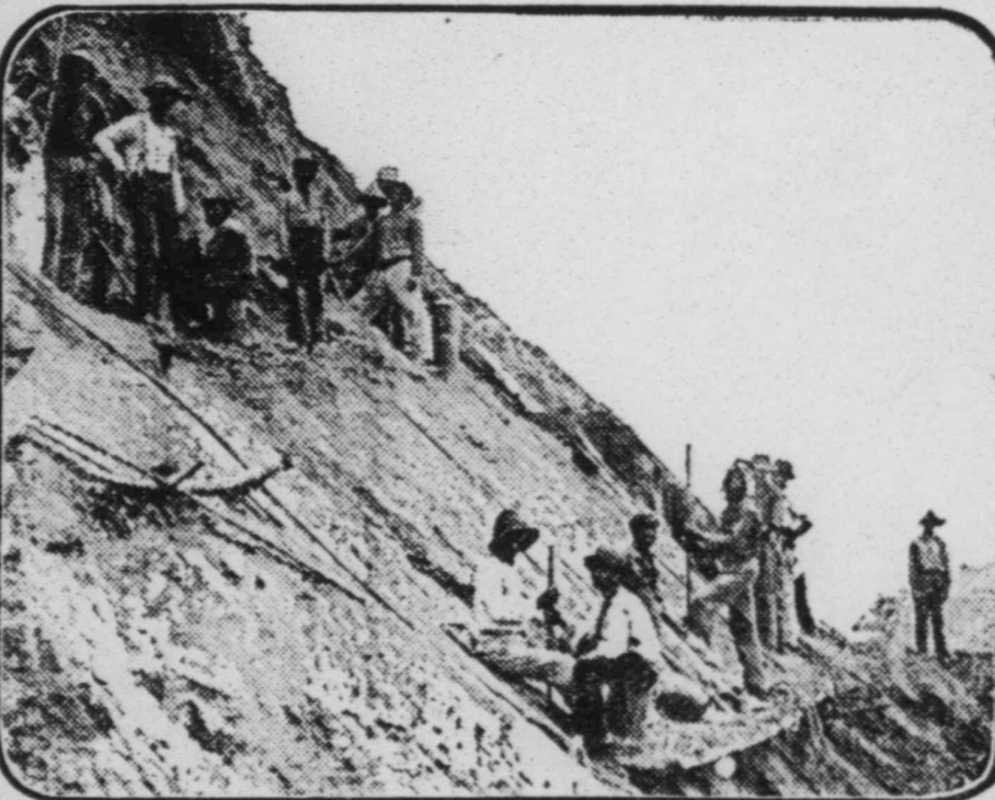
This picture shows the work of blasters on a big cut. The men are Jamaica negroes from Kingston. They get 10 cents an hour for ten hours per day. They usually put in about sixty shots a day and the fellow on top of
