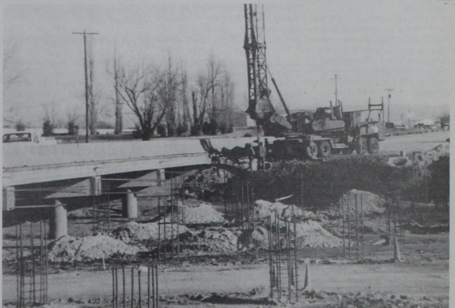
BRIDGE WORK (Not dental!)-Work continues on the widening of Highway 60 at the bridge over Frio Draw west of Friona, better known locally as the golf course bridge. Residents are hoping for a turn of good weather soon, so that more progress can be made on the highway widening project.
