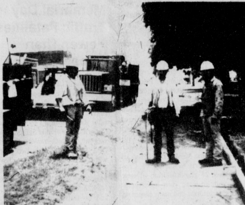
OLD SIDEWALK DEMOLISHED — Roadway Construction Company employees have demolished the old sidewalks in front of the First Baptist Church classrooms and are preparing for new ones.
