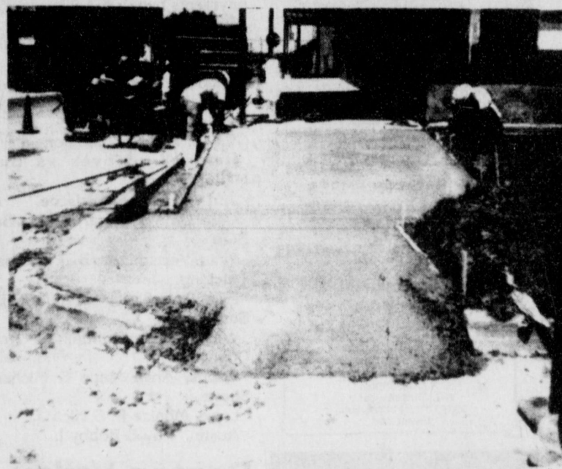
NEW SIDEWALK EXTENDING FROM HIGGINBOTHAM BROTHERS COMPANY — Employees of Roadway Construction Company attend to final details on the newly constructed sidewalk coordinated through TxDOT.
