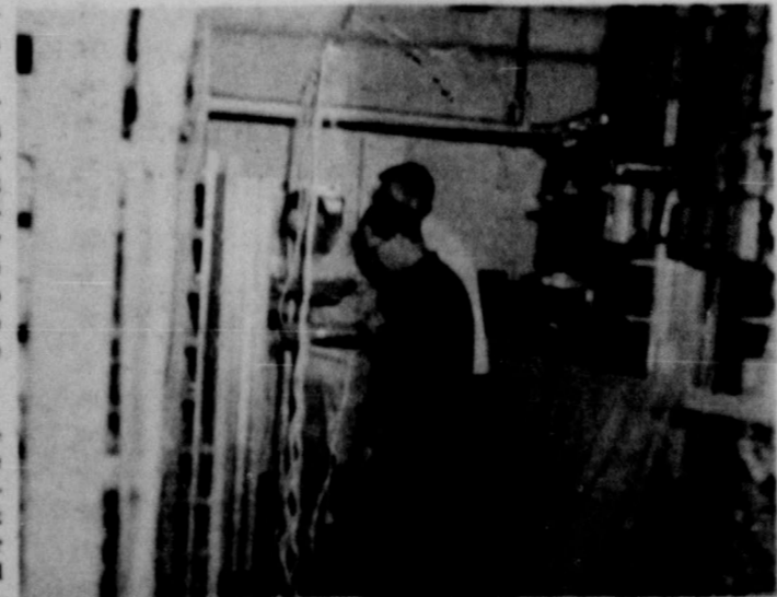
TELEPHONE EMPLOYEES are pictured pulling the cords that shut off the old switchboard and channeled a current to the new dial equipment. The changeover was made in a matter of seconds.
