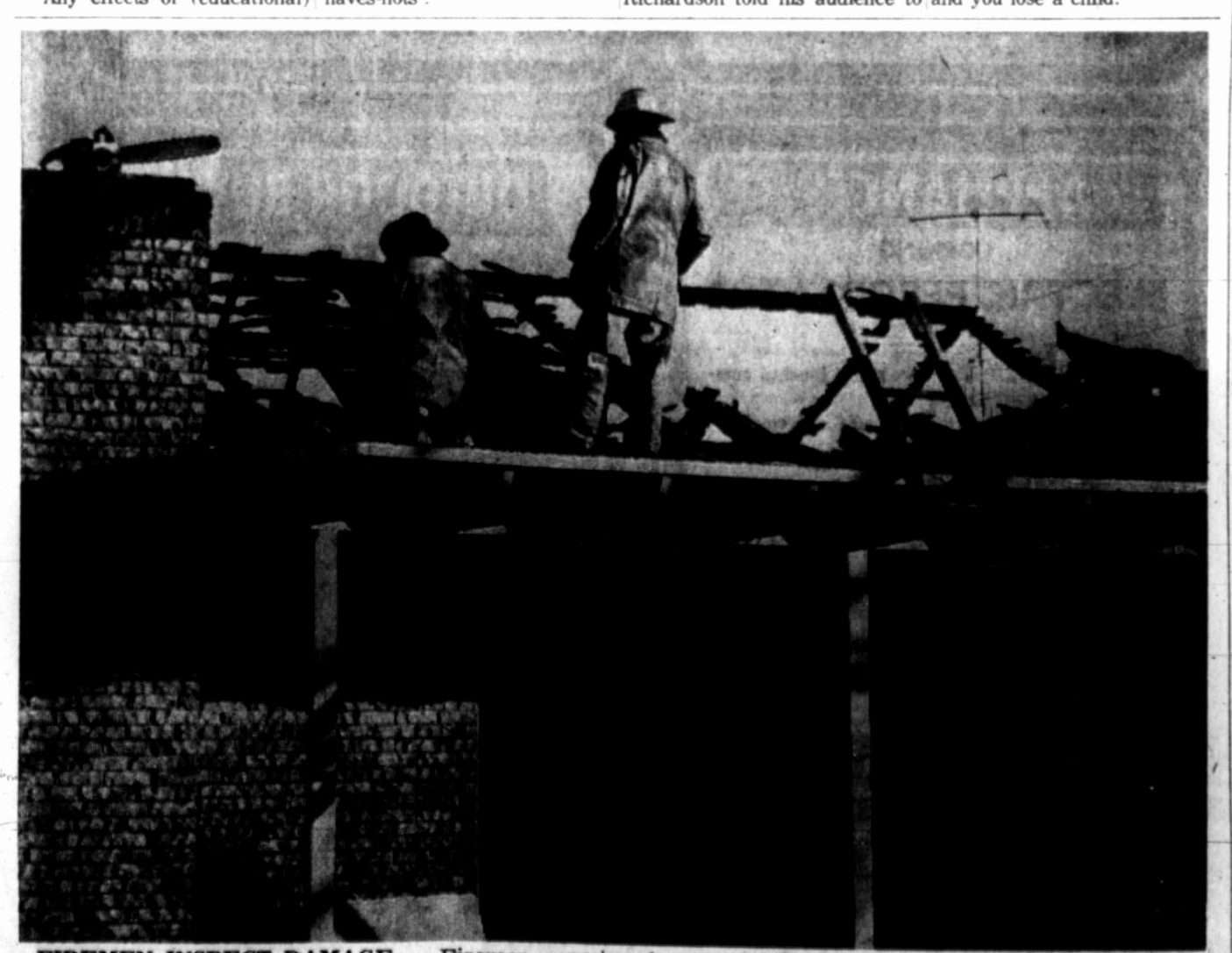
FIREMEN INSPECT DAMAGE — Firemen examine damage to the home of Dr. and Mrs. Royce R. Whitefield, 2601 Fannin St. An early-morning blaze caused heavy damage to the roof and ceiling of the home. Damage to the interior of the house was caused primarily by water and smoke. Reported at 7:43 a.m., the fire was under control within 30 minutes. The cause of the blaze is under investigation.
