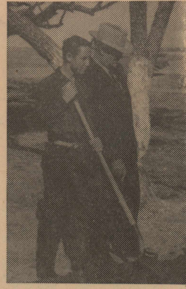
JOSEPH VANDERSTUCKEN, West Texas Boys Ranch director, observes Randy Miller of Odessa as he completes his part of a sidewalk project. Randy is receiving special vocational training in addition to his regular academic work. He and a special crew recently completed pouring sidewalks at the Ranch.
