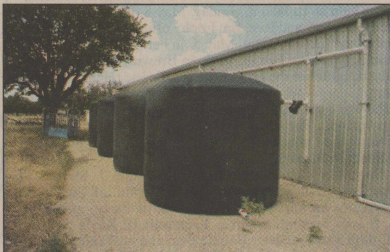
The 3,000 gallon storage tank serves as the backbone to the Condrarosa's water harvesting system.
