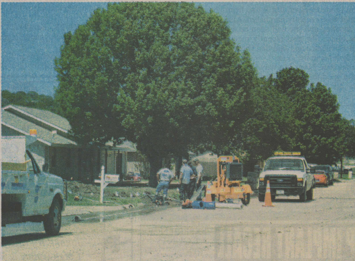
City of Sonora employees battle a mainline water leak on Deerwood Street on Friday March, 30th.
