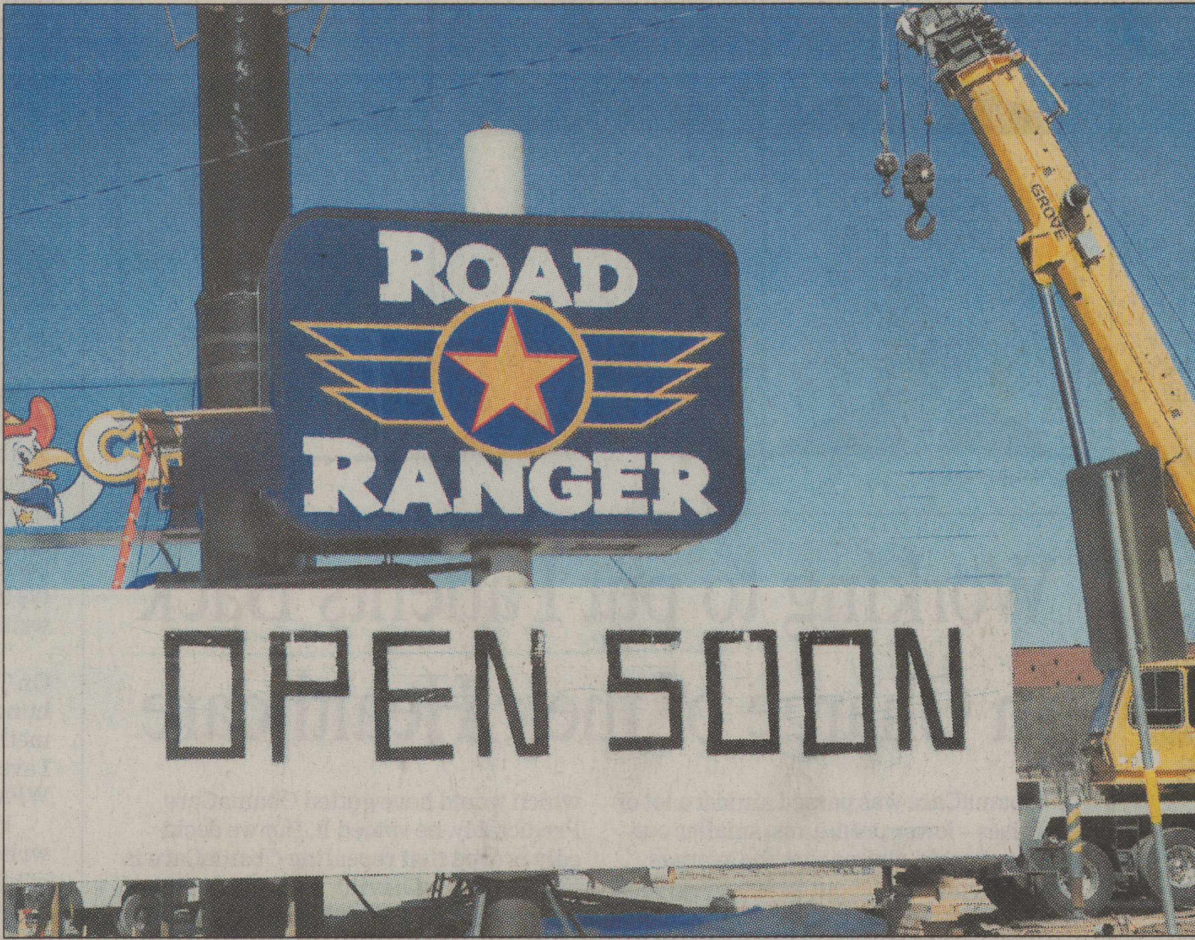
Construction continues on the new Road Ranger Travel Center located at the I-10 and Hwy 277 exchange in Sonora. The new facility will include a Chester's Chicken and Texas Taco restaurants. KIMBERLEY MEYER | THE DEVIL'S RIVER NEWS
