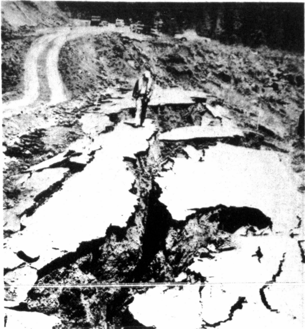
STATE HIGHWAY Engineer Harry Apodaca walks along a section of New Mexico highway between Jemez Springs and Los Alamos that collapsed in mud due to a heavy spring runoff. The road sank during a 48-hour period Tuesday and Wednesday.
