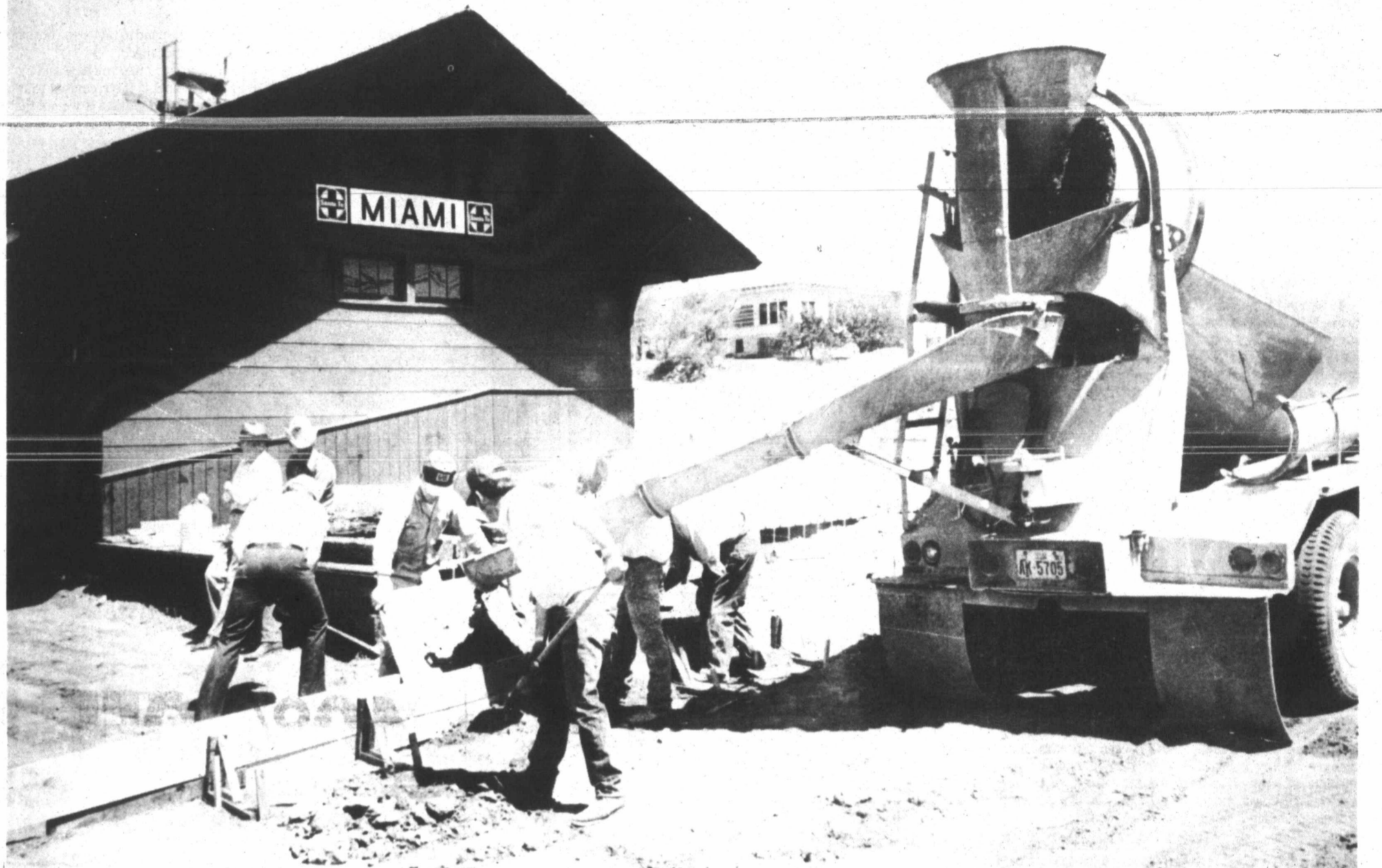
WORKMEN pour concrete around the Roberts County Museum. The museum, which is scheduled to open June 2, will be the main attraction during the Miami Cow Callin' contest. (Staff Photo)
