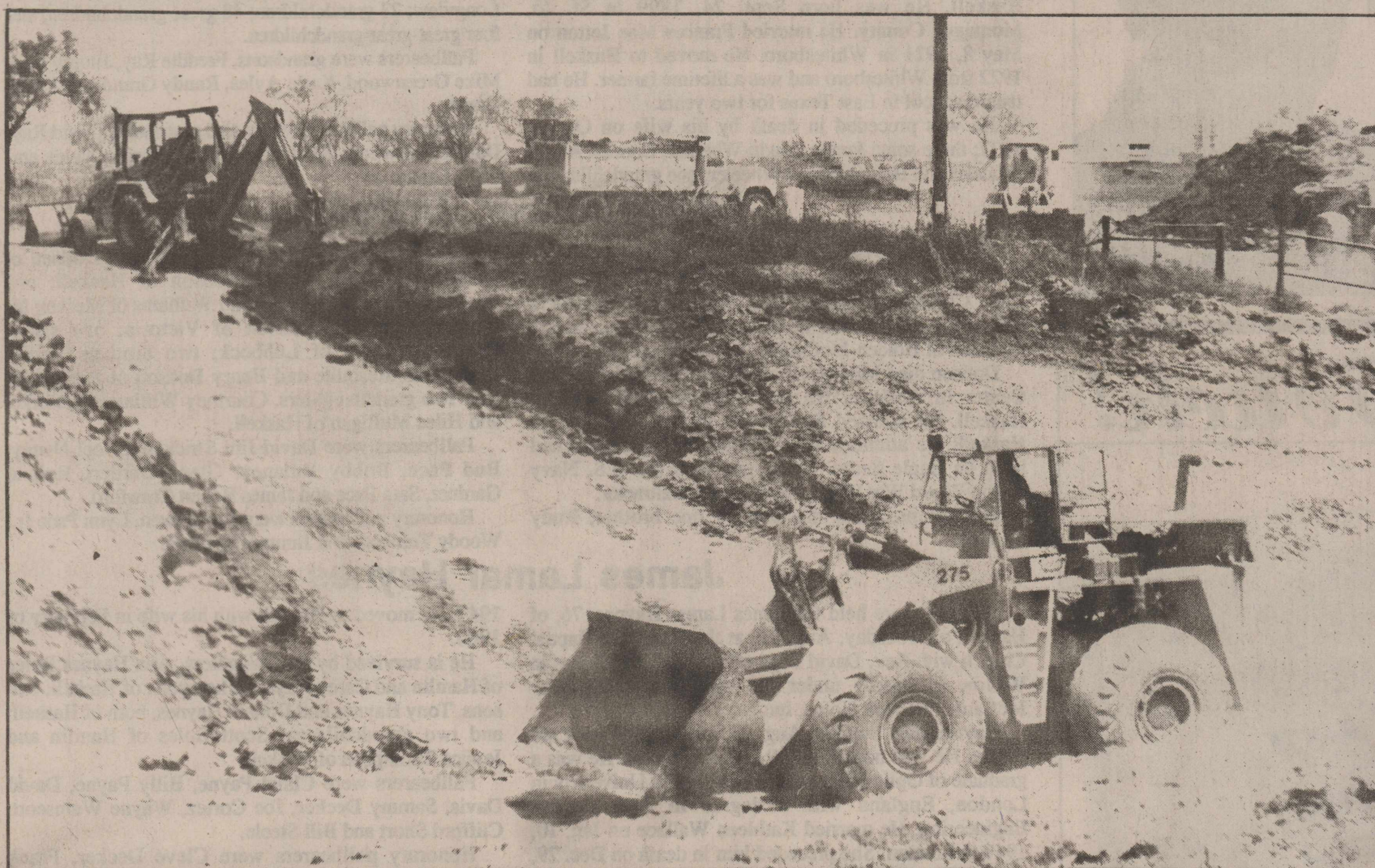
DREDGING OUT A NEW BOAT CHANNEL - Heavy equipment operators have been busy at Scott Memorial Park, dredging out a new boat channel, and a location for a concrete ramp and a boat dock while the water in the lake is low.
