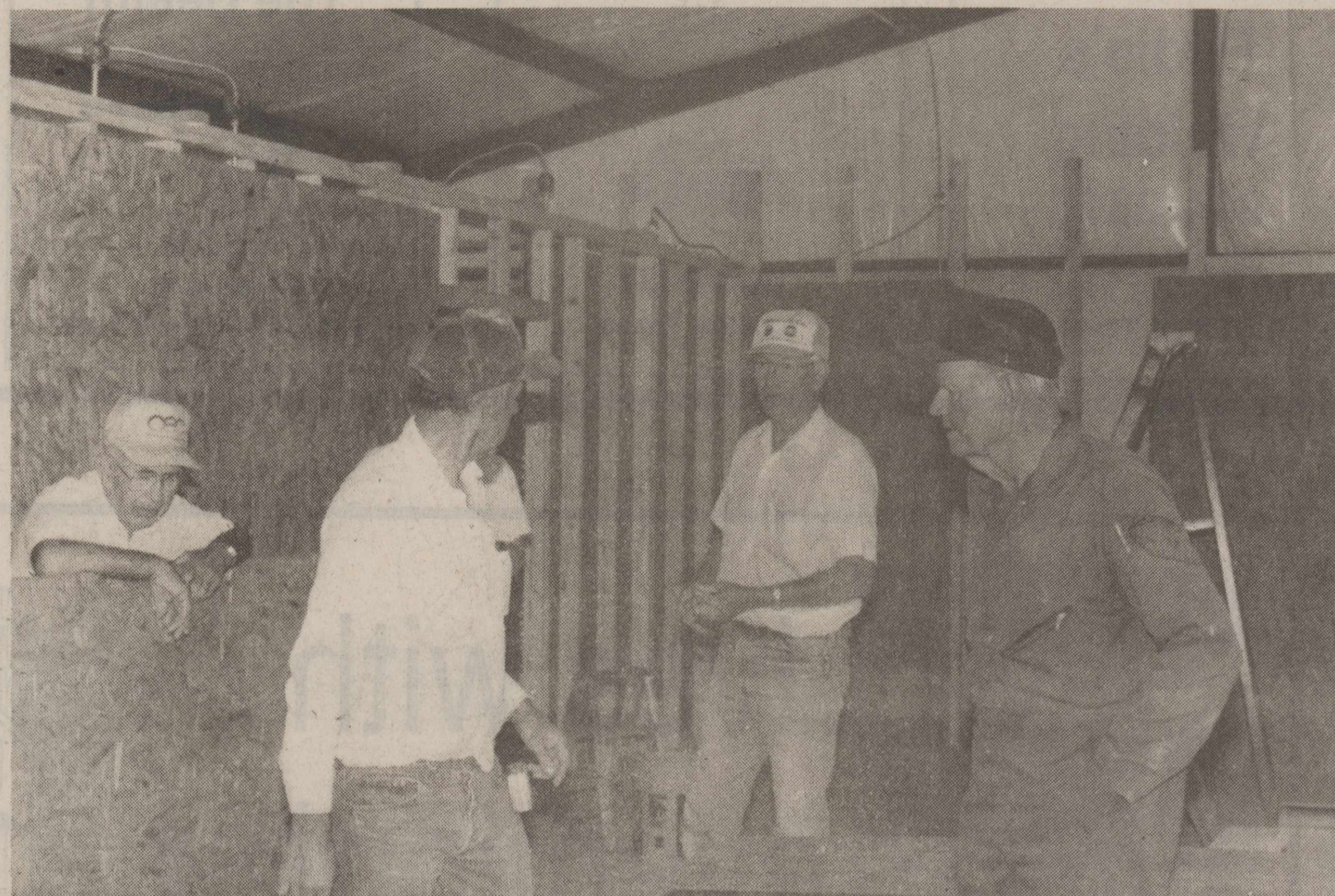
MEN ON A MISSION — Local Baptist men Virgil Cobb, right, Ronnie Chapman, Troy Culpepper and R. V. Earles worked recently on the Fellowship Hall being constructed at the Calvary Mission. Others helping with the project were Jim Turner, Bob Aycock, Wayne Waincott, Earl Smith, Derek Osborn, Ford Cole, George Fouts and Milton Christian. Ladies from Calvary Mission prepared lunch for the workers.
