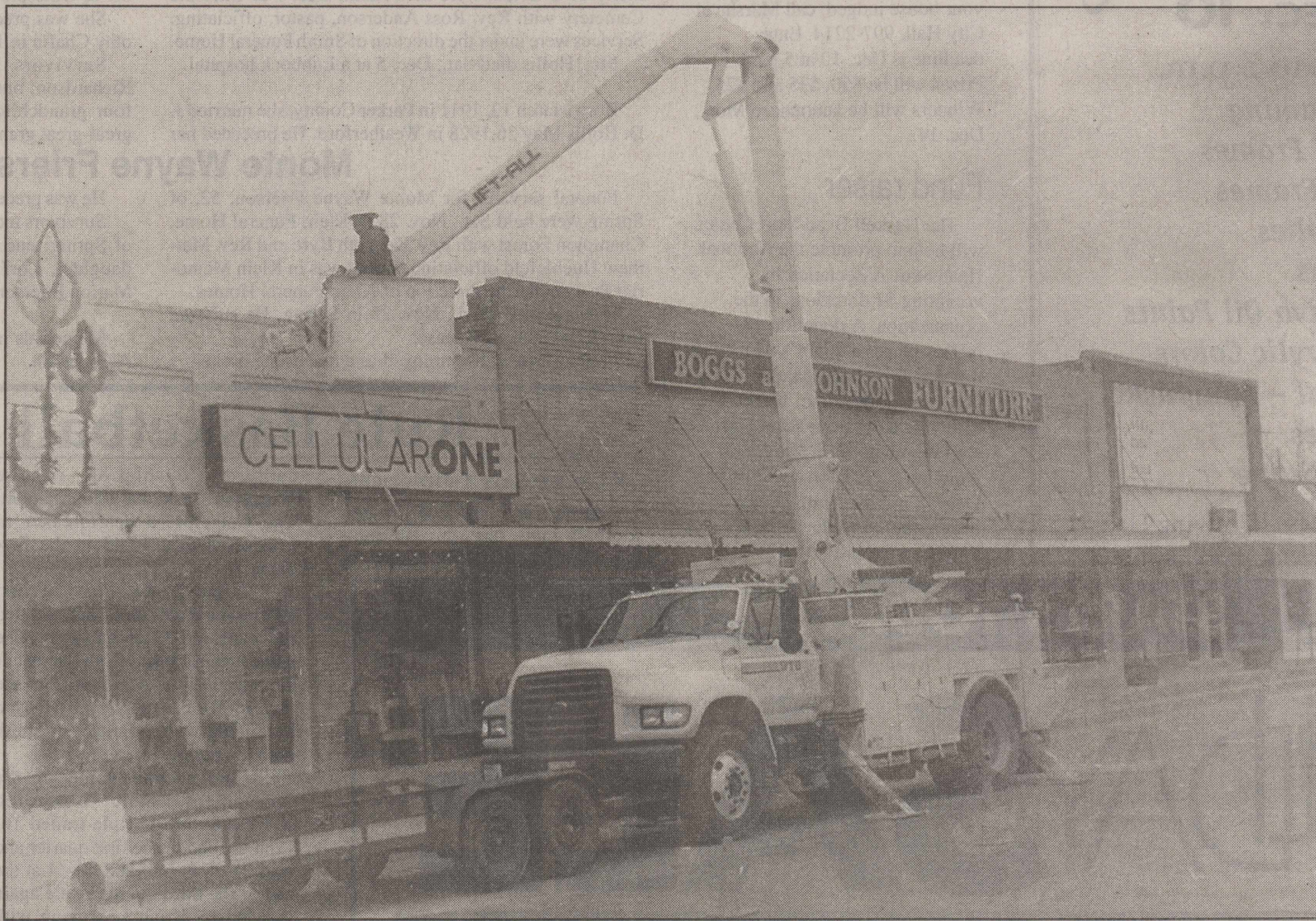
LIGHTING UP —Crews from West Texas Utilities were helping to install the downtown area Christmas lighting early this week.
