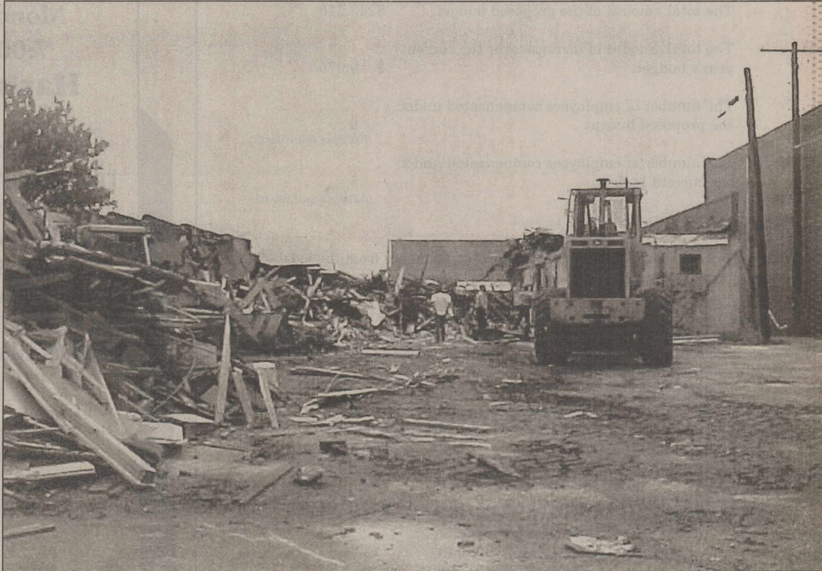
MAKING WAY FOR PROGRESS -Demolition crews began work on the first phase of work planned for clearing away old buildings
