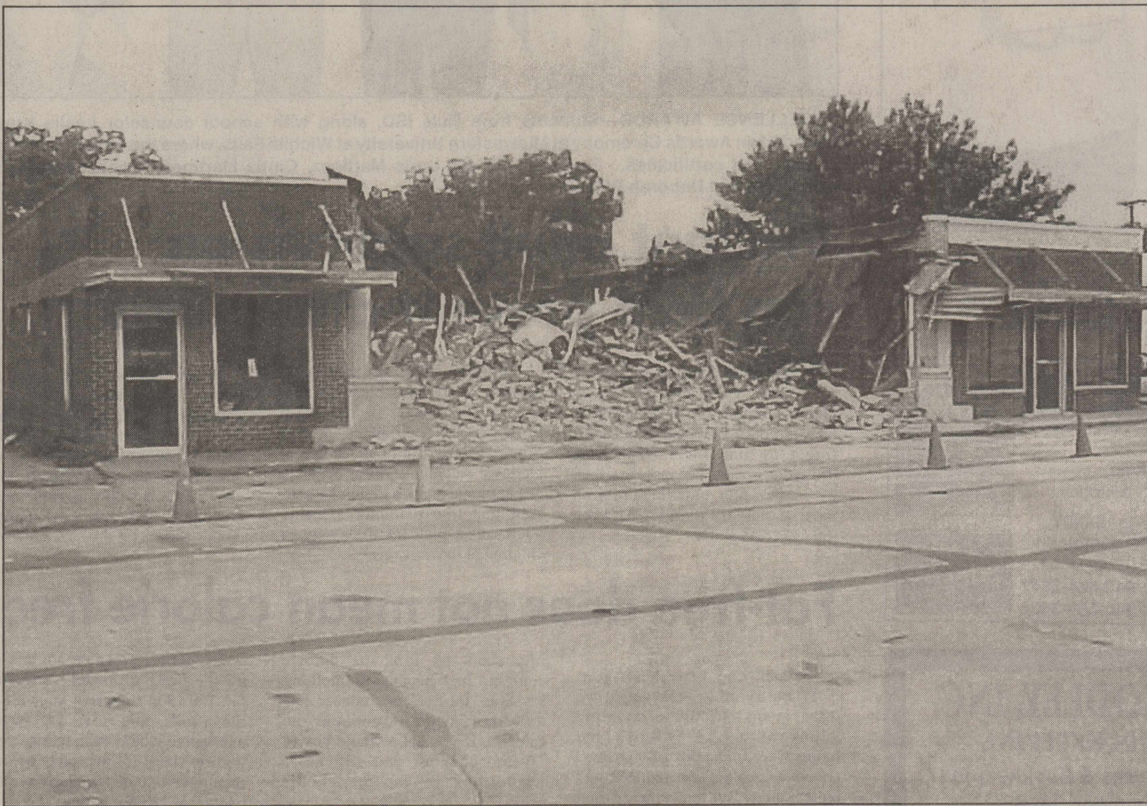
THE WALLS CAME TUMBLIN' DOWN -Work continues this week on the demolition of old buildings located on the west side of the 100 block of North Ave. E. in downtown Haskell. The City owned lots are being cleared to make room for future development.
