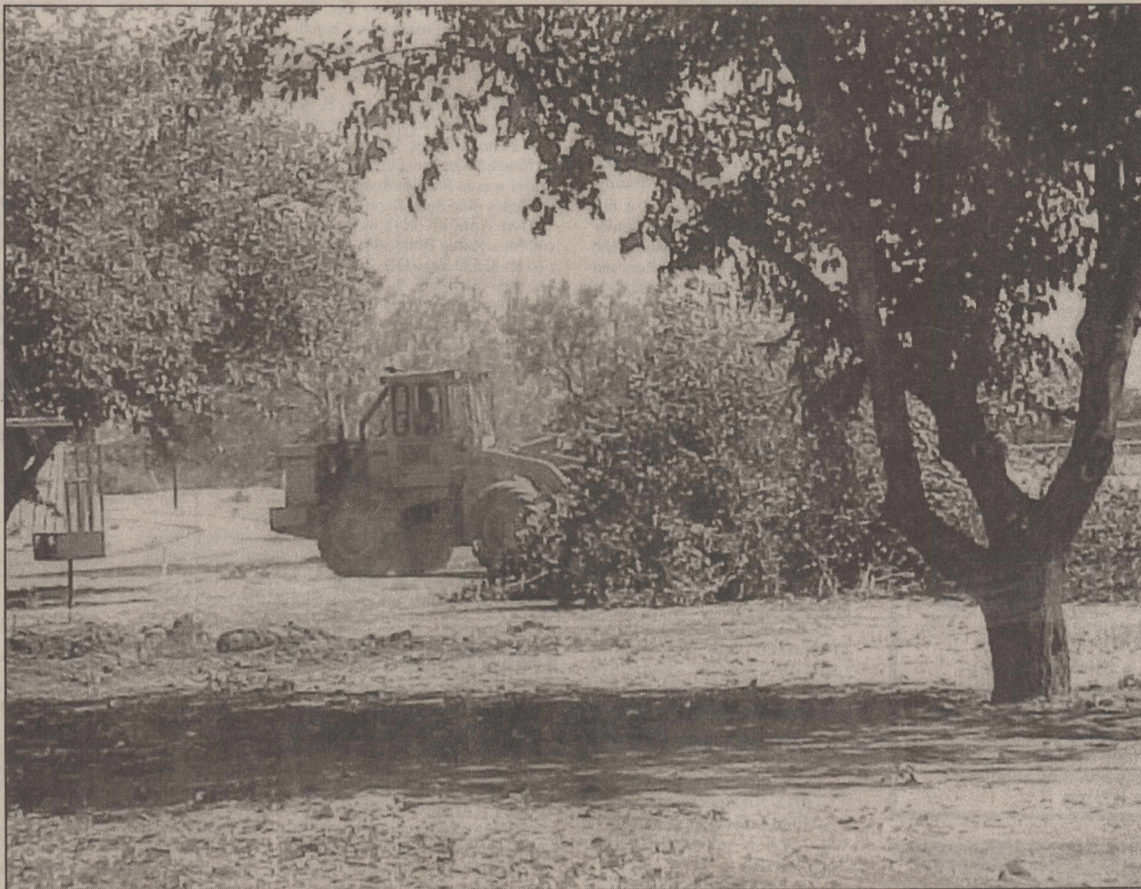
MORE ROOM FOR HAPPY CAMPERS —City of Haskell crews this week began clearing space for additional camper hookups for
