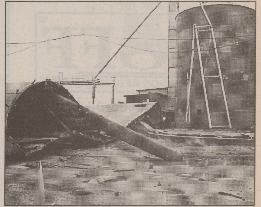
Grain bin at former Haskell Grain location, S. First and Ave. A
