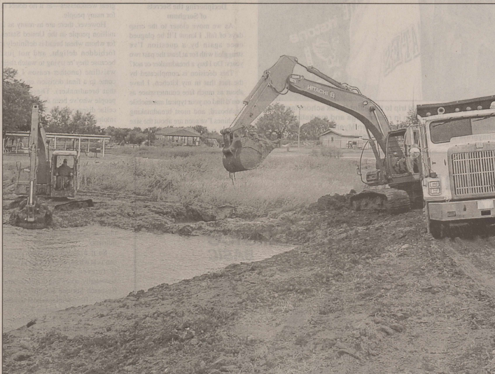
CREEK CLEAN UP BEGINS —Equipment began working on the clean up of Rice Springs Creek this week. Two track loaders and three dump trucks are at work on the project consisting of de-
