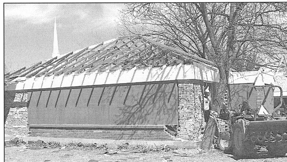
OLD LIBRARY RAZED —Jim McTasney, standing in the doorway, is disassembling piece by piece the old library building located at 300 N. 1st in Haskell. A new library is planned for the location.
