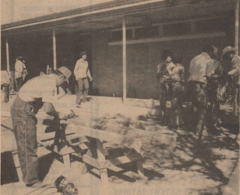
PLAYGROUND EQUIPMENT GETS INSTALLED at Ozona Primary School Saturday. The new playground equipment was a project of the Ozona Womans League. League members prevailed upon husbands and youngsters to assist with the project and after an all-day workout the equipment was ready for use Monday morning.
