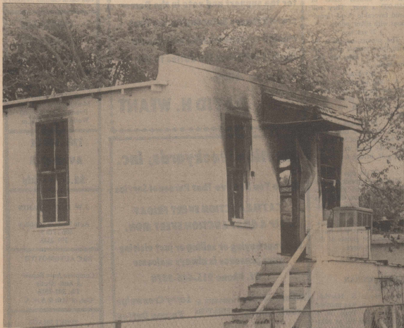
GAS EXPLOSION Friday morning at 606½ Ave. G in a garage apartment sent a couple to the hospital with burns and the resulting fire gutted the inside of the apartment. The explosion knocked the walls off center and blew the
