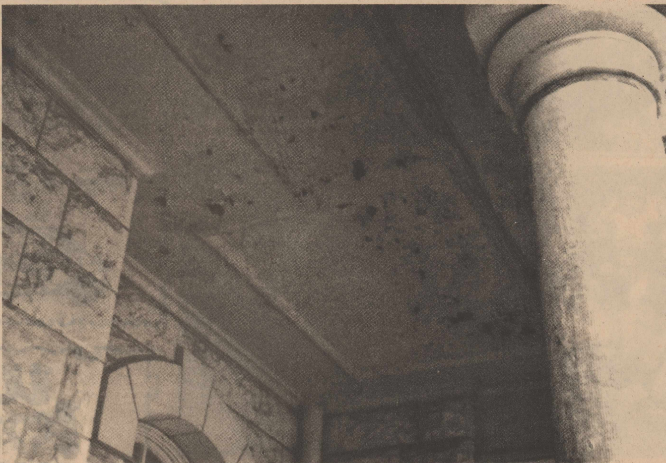
COURTHOUSE IN DIRE NEED OF REPAIR -An inspection of the courthouse, both inside and out, revealed what a shocking lack of maintenance and upkeep the building has suffered. Here the paint peels off the tin ceiling and rust has taken over.
