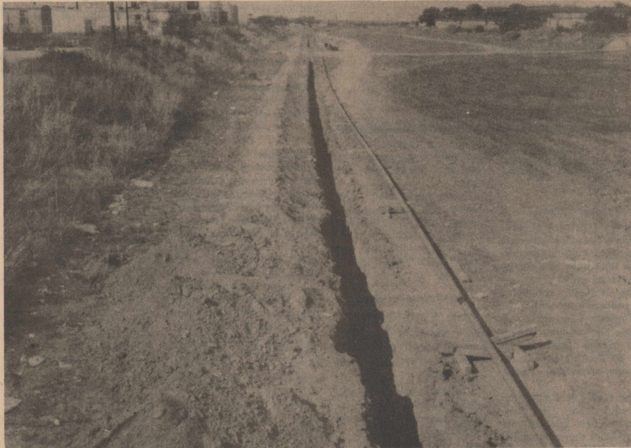
OIL GOES UP, WATER COMES DOWN in Johnson Draw. Final drainage of flood waters through Ozona, Johnson draw figured in the Soil Conservation Service's Ozona flood control plan after the 1954 flood and now furnishes the right of way for an oil pipeline carrying oil or gas from a town well
