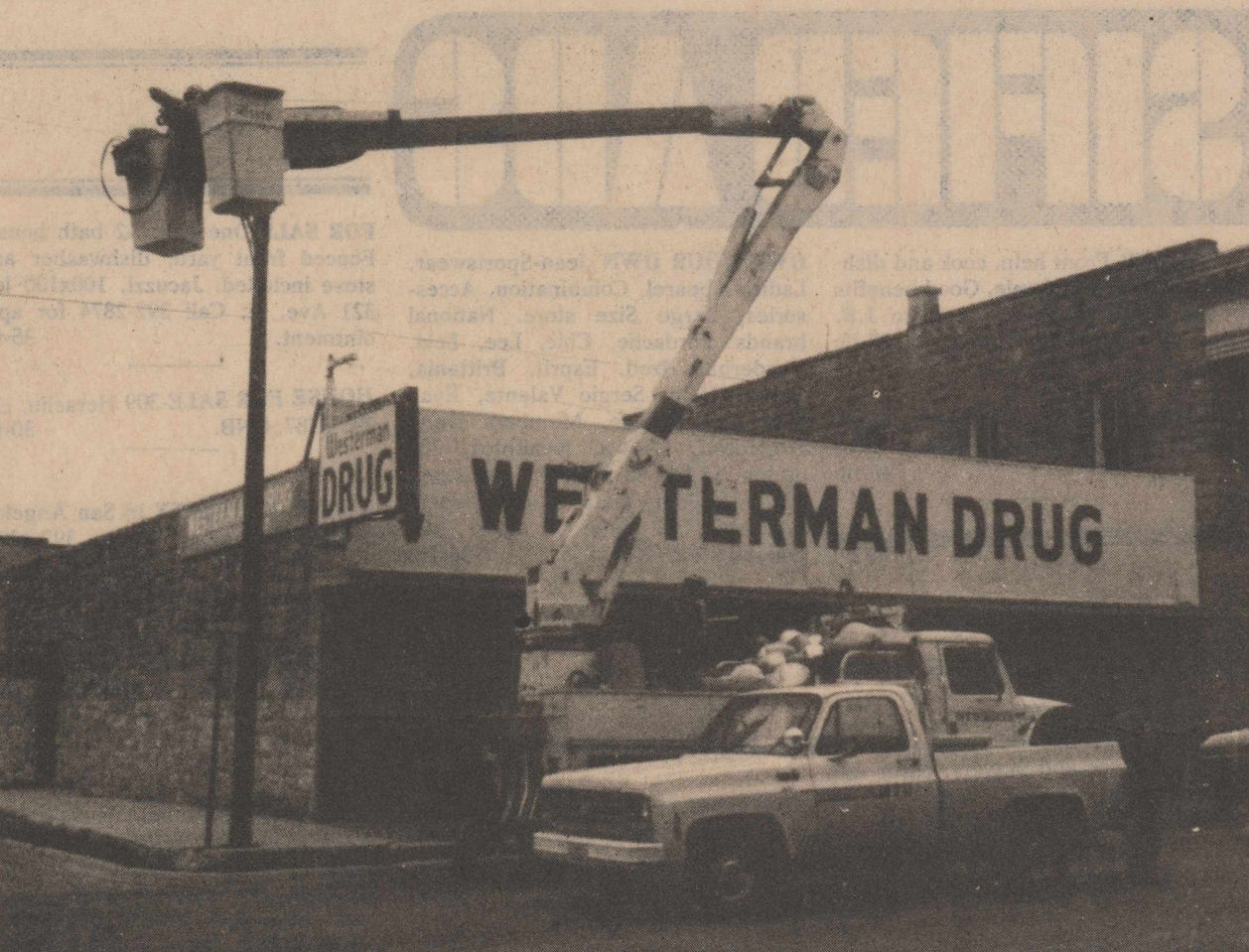
New energy-saving lights
